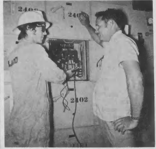
Employee Harry Koolman (r) observes student Efrain Kelly at work here in the NFAR switchroom.
